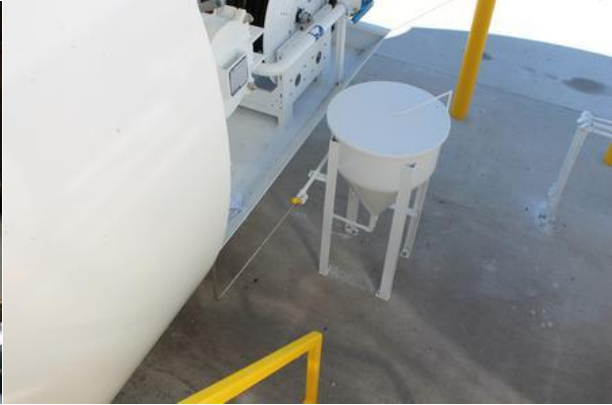
Sump Fuel Recovery Unit, Winter Haven, FL
